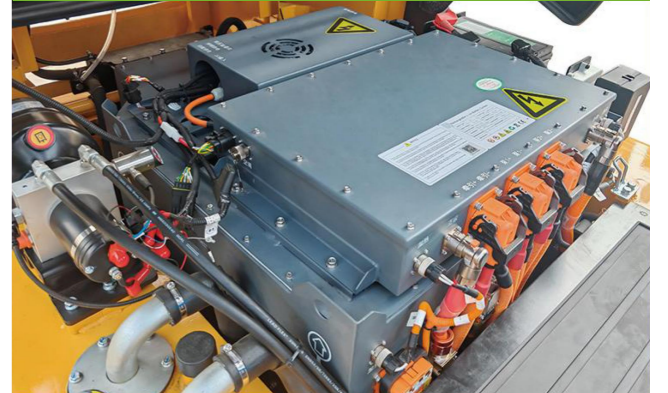
Large capacity lithium battery(max.81.6KWh)
