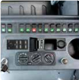
Centralized Instrument Switch Panel
